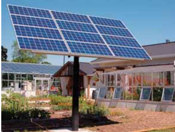
Solar Array at SENS House
